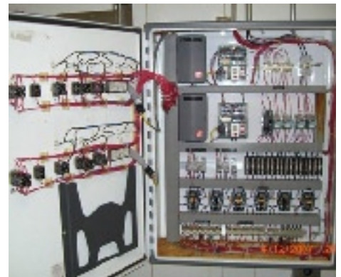
Modifying the electrical controls for the evaporator fans saves $7,000 annually.
