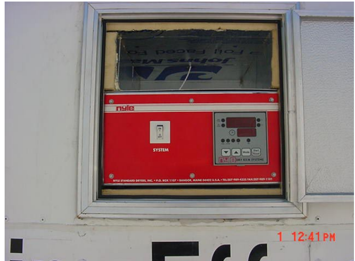
Figure 4. Control Unit Accessible from Outside of Kiln
